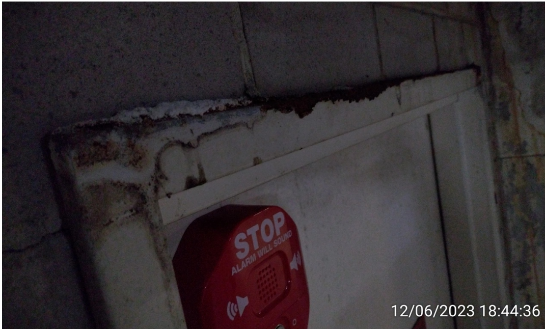
Fire door in basement of Block D:
