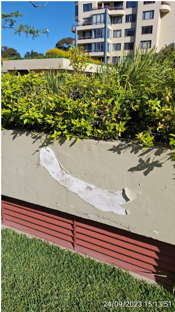
Examples of garden bed damages:
