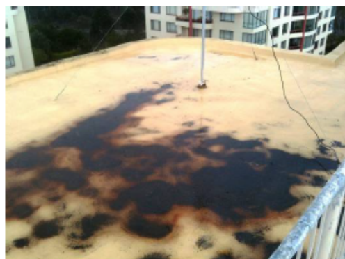
Standing water to flat roof deck, Block A
