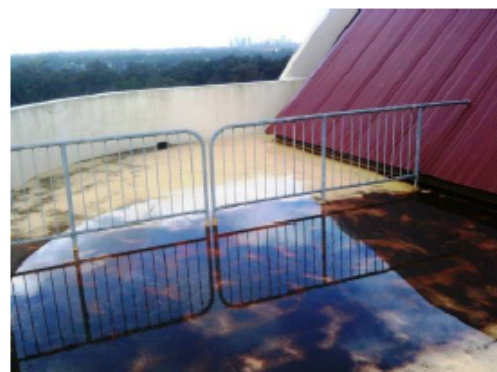
Standing water to flat roof deck, Block B
