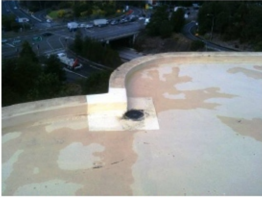
Previous patch works evident
