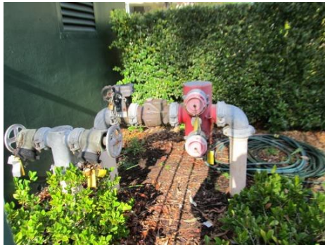
Hydrant booster connection
