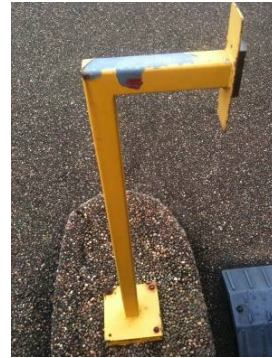
Redecoration required to metal surfaces
