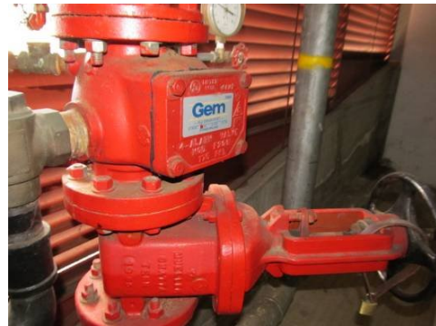
Sprinkler valve set
