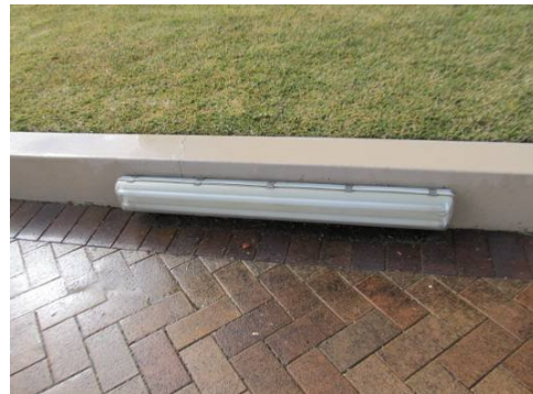
Typical exterior lighting
