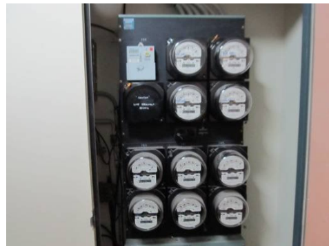
Typical tower residential units authority meters
