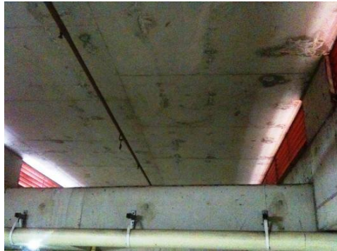
Minor water penetration through soffit
