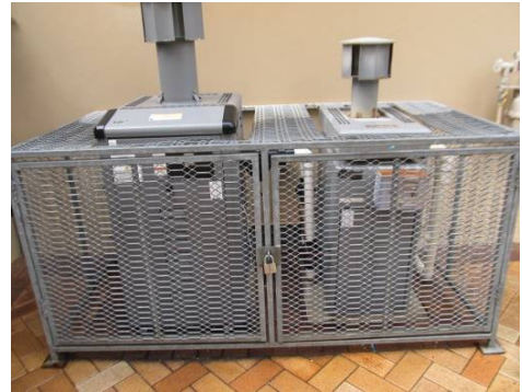
Gas fired swimming pool and spa heaters
