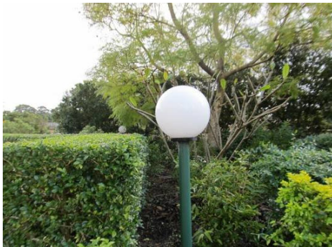
Typical common area garden lighting
