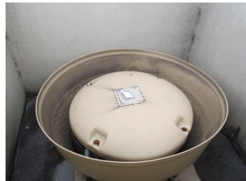
Typical unlabelled roof mounted fan
