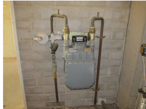
Typical gas meter in the tower building boiler rooms
