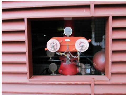
Sprinkler booster connection
