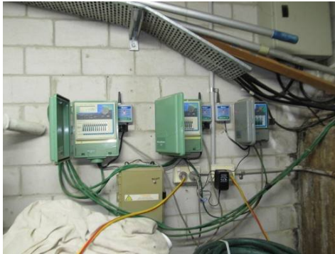
Automated controls for the garden irrigation system
