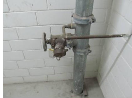
Typical tower building hydrant land valve
