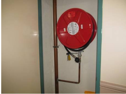
Typical tower building hose reel
