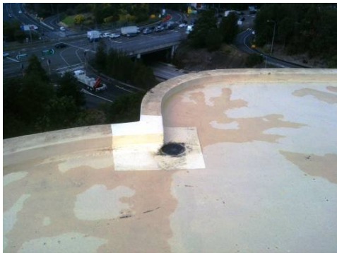
Previous patch works evident
