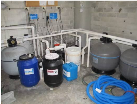
Swimming pool and spa filtration systems
