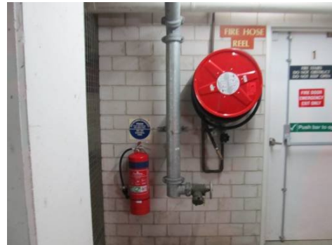
Typical car park extinguisher, hydrant and hose reel
