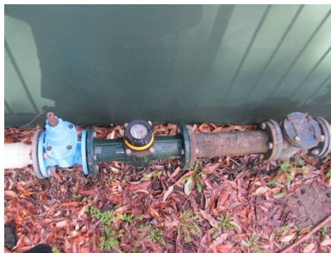
Authority water meter without back flow prevention device installed
