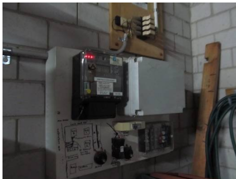
Common area authority meter
