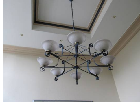
Typical tower main lobby lighting
