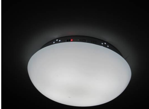
Typical tower building new common area lift lobby lighting
