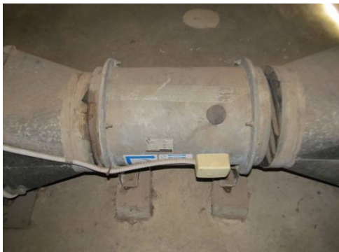
Typical unlabelled Inline axial fan located in roof top plantroom
