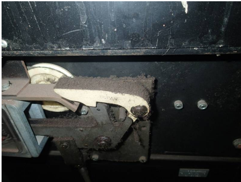
All lift shaft equipment must be cleaned
