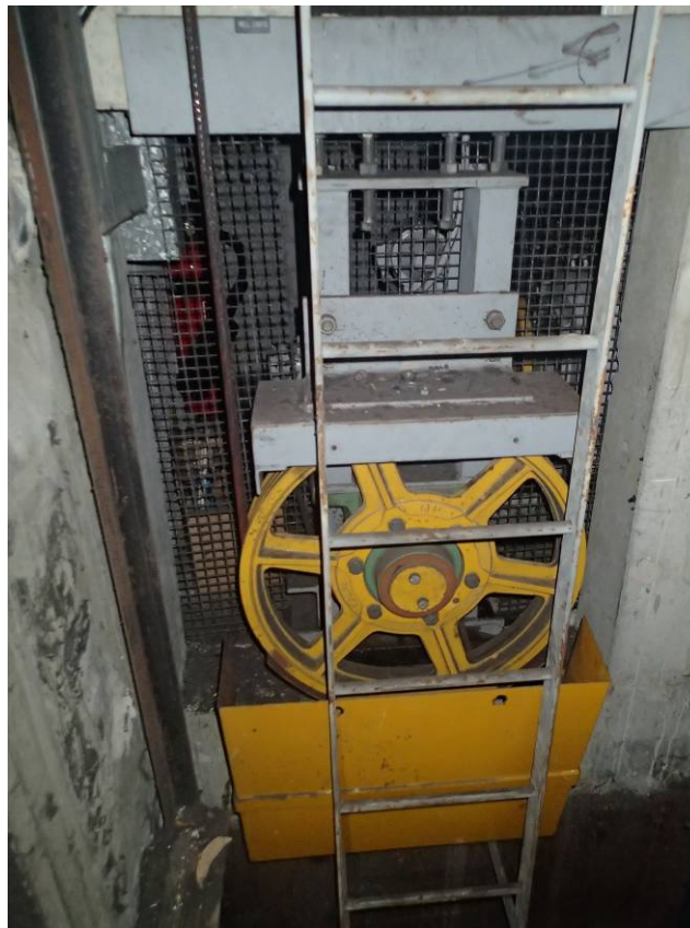
Traction sheave guards must be correctly installed
