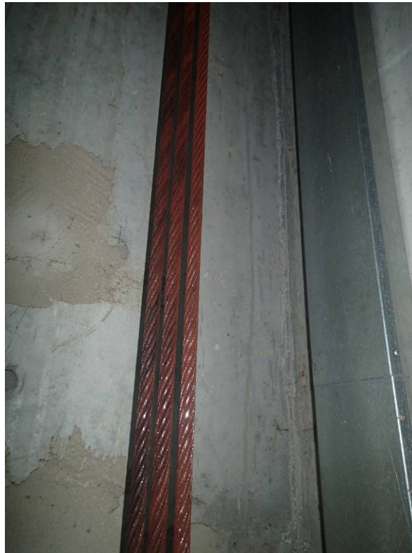
Rusty hoisting ropes must be replaced
